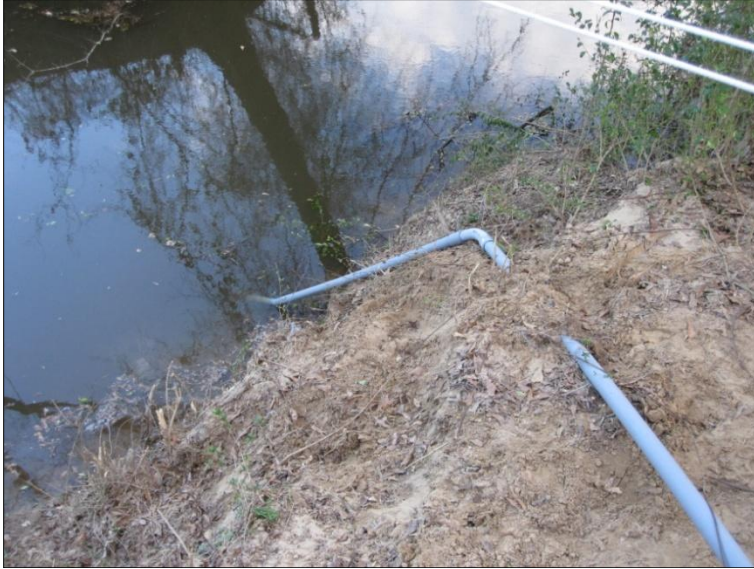
Figure 19 Submerged pressure sensor probe incased in perforated PVC
