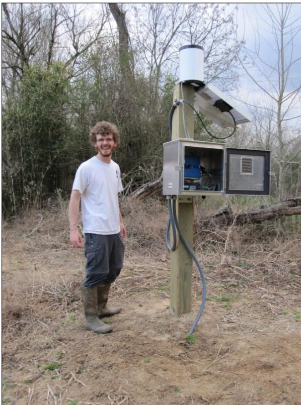
Figure 18 Rain gauge, interface module, battery, and solar panel
